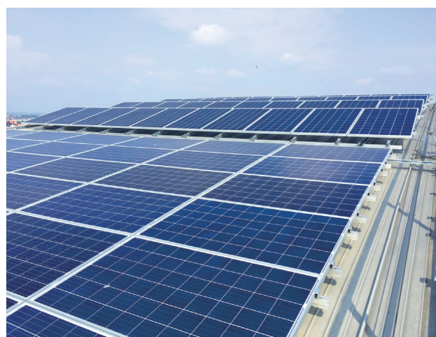
Westquay photovoltaic array
