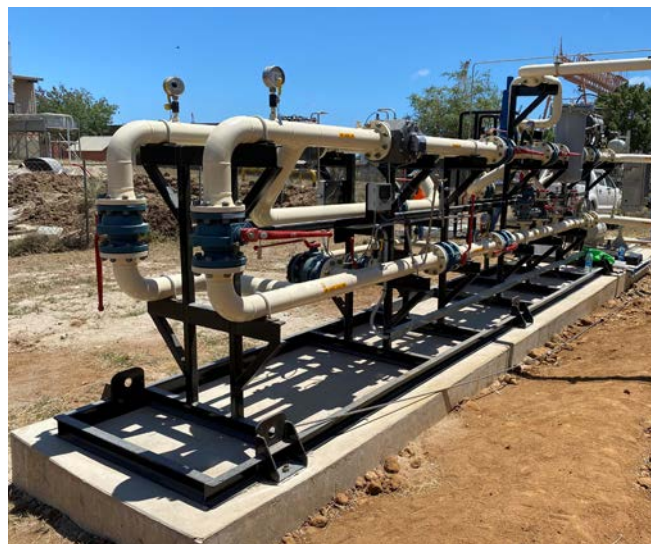
Metering skid and odorizer at the GRF at Mtwara
