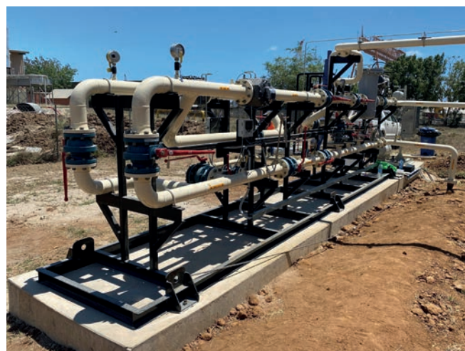
Metering skid and odouriser at the GRF at Mtwara
