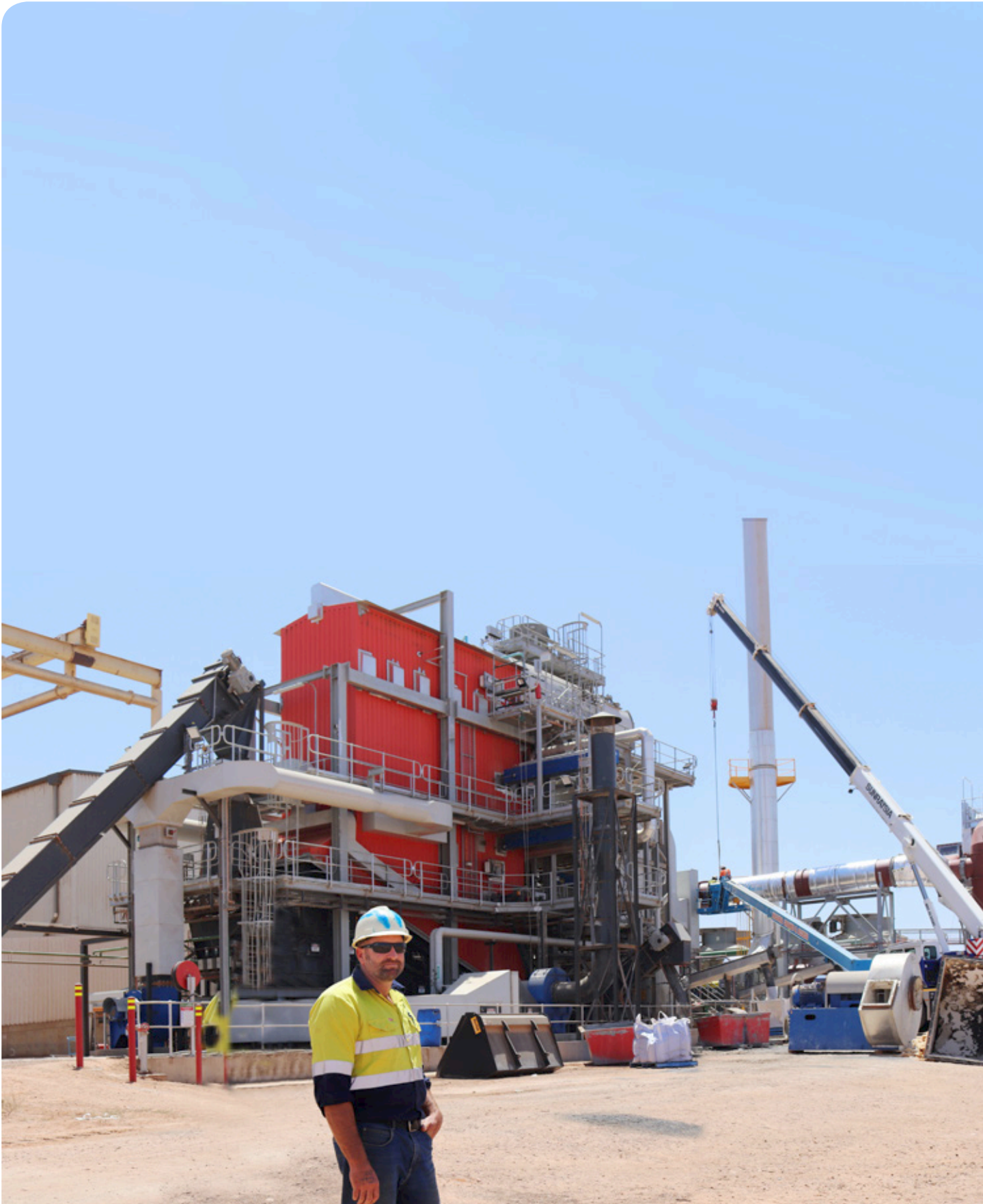
ABOVE: Daniel Wilson, H2E Operations Manager, overseeing installation of the H2E bag filter
