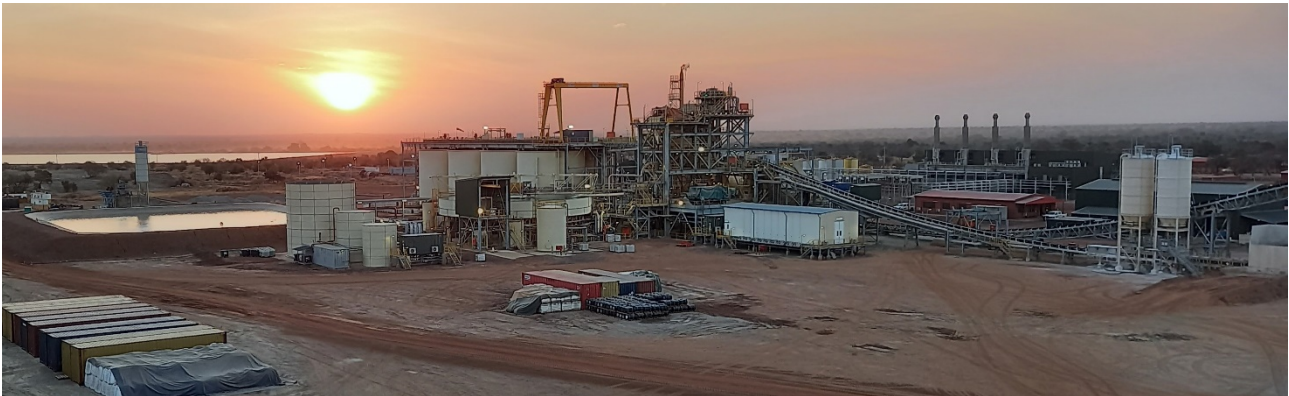
figure 1 - Sanbrado processing plant
