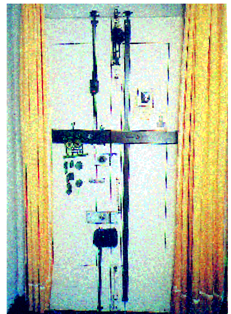
More security does not always mean higher security, if the product is not user-friendly. More security may even make it difficult to evacuate the premises, as in this apartment in Genoa, Italy.
