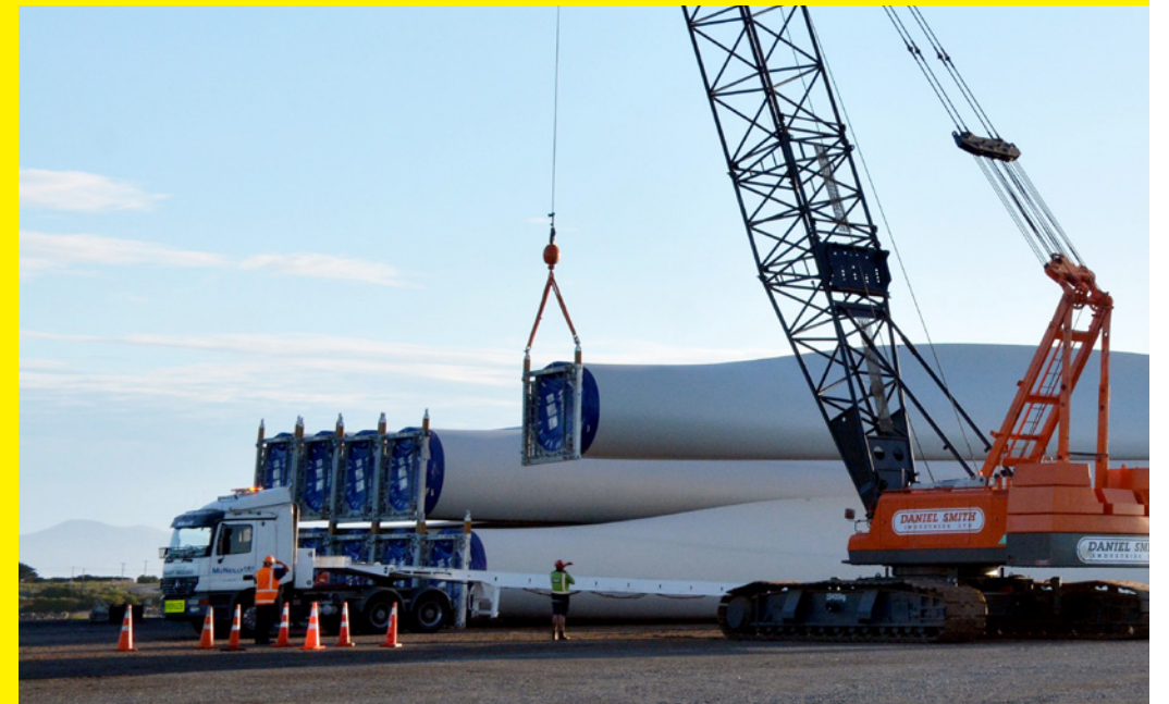
Blades for the turbines at Kaiwera Downs 1 wind farm unloading at Bluff - credit South Port, Chris Howell.
