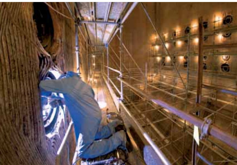
Pictured above is the inside of Unit #2's boiler at Stuart Station. When the unit is operating, temperatures inside the boiler reach 2,500 degrees Fahrenheit.
