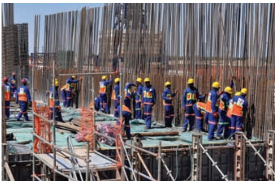
The product screening facility under construction at Kumba Iron Ore's Kolomela project. The mine is on schedule to start production in the first half of 2012, ramping up to full capacity of 9 Mtpa in 2013.
