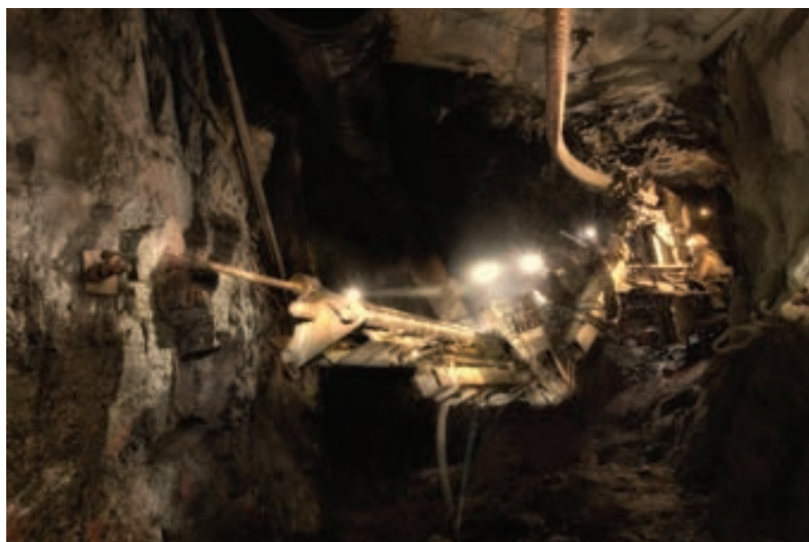
Hydropower equipment (HPE) raise rig drill at Twickenham Mine. HPE forms part of Anglo Platinum's mechanisation programme which is leading to higher quality raise development than through using conventional drilling and blasting, and faster rates of development, as well as safety benefits as fewer employees are needed in the critical drilling areas.
