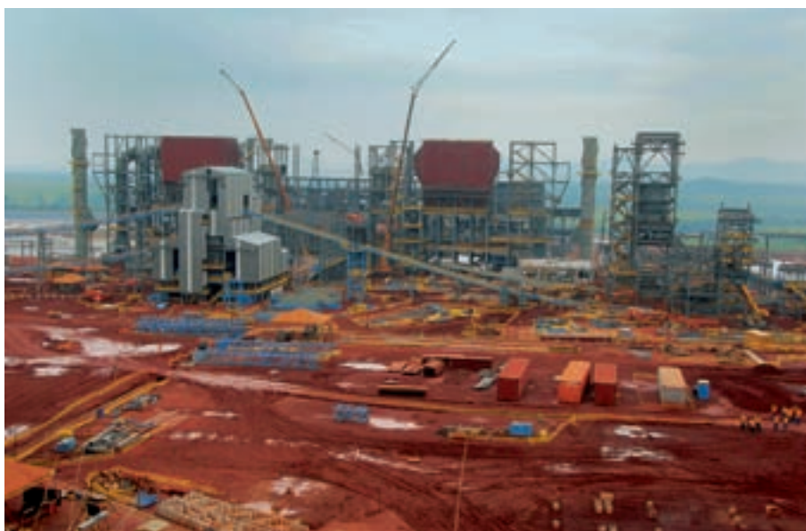
Construction work on the ferronickel plant at the Barro Alto project, which is due to produce its first metal in 2011, ramping up to an annual production of 41 kt over the first five years of a forecast 25 year life.
