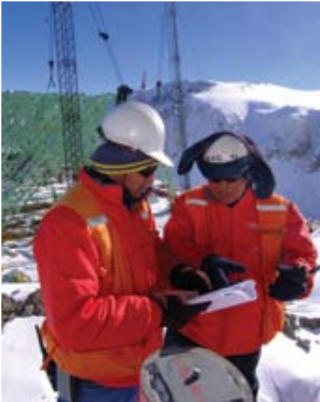
The Los Bronces copper expansion project in the Chilean Andes is due to come on stream in the fourth quarter of 2011.
