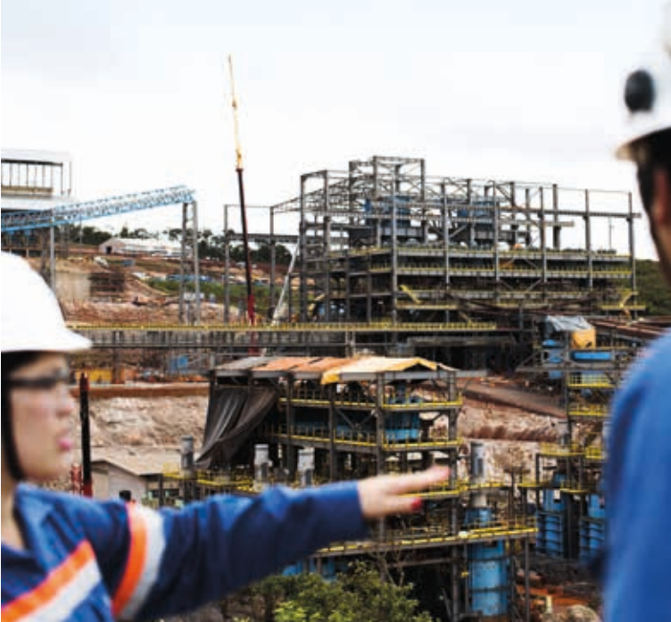
Image Construction work at the mine site of the Minas-Rio iron ore project. By year end, the project was 84% complete overall, with the beneficiation plant 83% complete and the 525-kilometre pipeline almost fully assembled.
