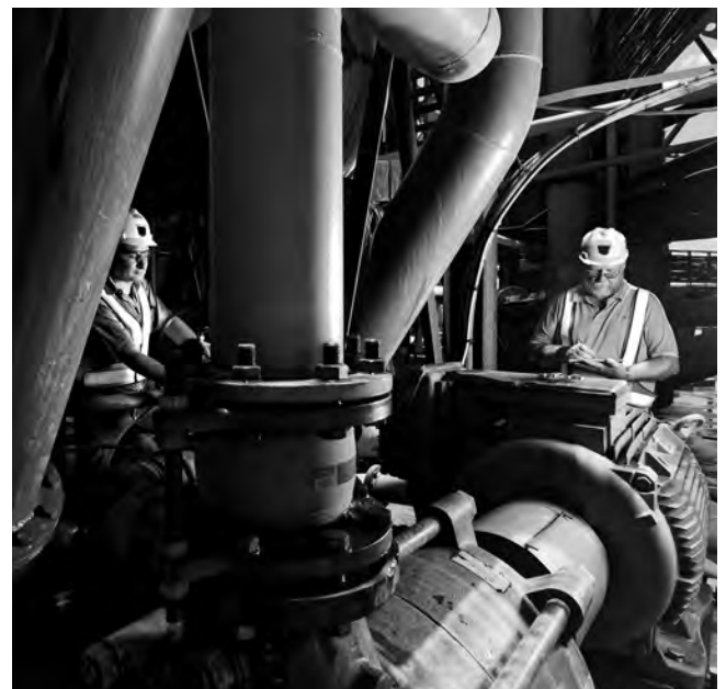
Asset manager Willem van Loggerenberg (left) and fitter Hendrik Landsberg recording data at one of the ore-slurry pumps at the concentrator at Amandelbult, a mine which, unusually, has both underground and opencast operations.
