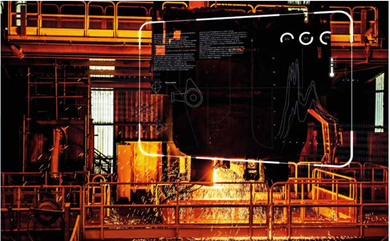
Predictive maintenance technology, which forms part of our FutureSmart Mining™ programme, is deployed at Barro Alto, where two electric furnaces are monitored by data platforms for performance levels and to detect maintenance needs.
