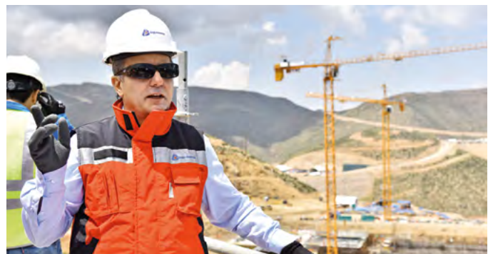
⤵ In March 2020, Marcelo Bastos stands at the place where the final stockpile dome will be constructed at the Quellaveco copper project.
