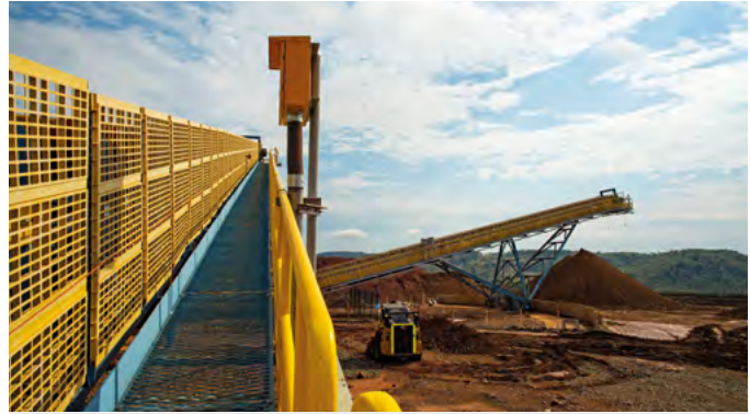
⤵ The bulk ore sorting (BOS) facility at our Barro Alto nickel operation in Brazil. The primary benefit of the BOS system, which has wide potential applicability across our business, is in unlocking capacity in the mining value chain through the early rejection of waste material.
