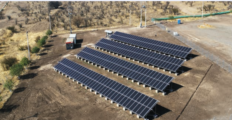
▲ At our Las Tórtolas site, which forms part of Los Bronces mine, we are making history by commissioning the first facility in Chile to generate 'green' hydrogen for carbon-zero vehicles. The plant will produce hydrogen from re-used water from the mining and treatment processes, and from photovoltaic (PV) energy sources, and represents an important step in our business's journey towards achieving carbon neutrality by 2040.
