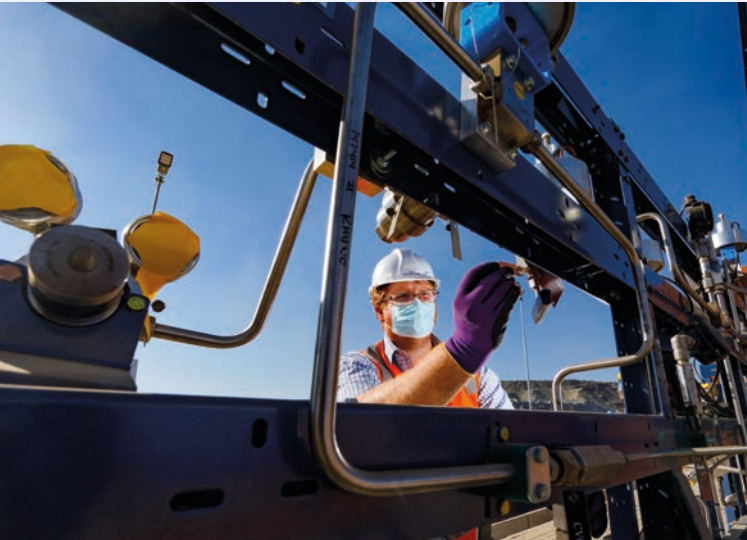
▲ Power engineer Carl Van Den Ordell makes adjustments to equipment during the construction of the hydrogen plant at our Mogalakwena PGMs mine.
