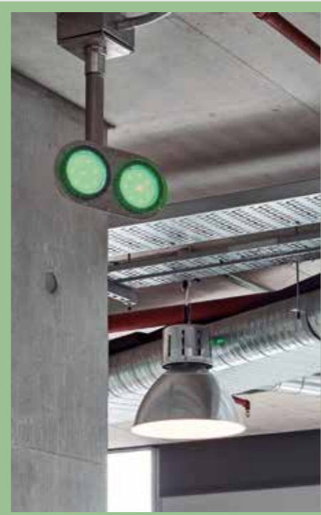
Above: White Collar Factory EC1: Traffic light building management system to denote windows are openable to allow for natural ventilation
