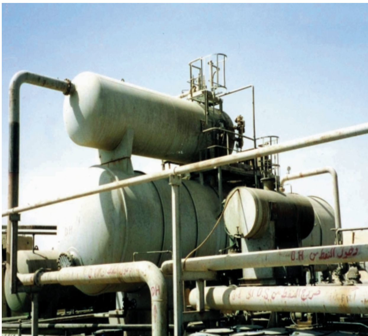
Luhais Existing Separator Units
