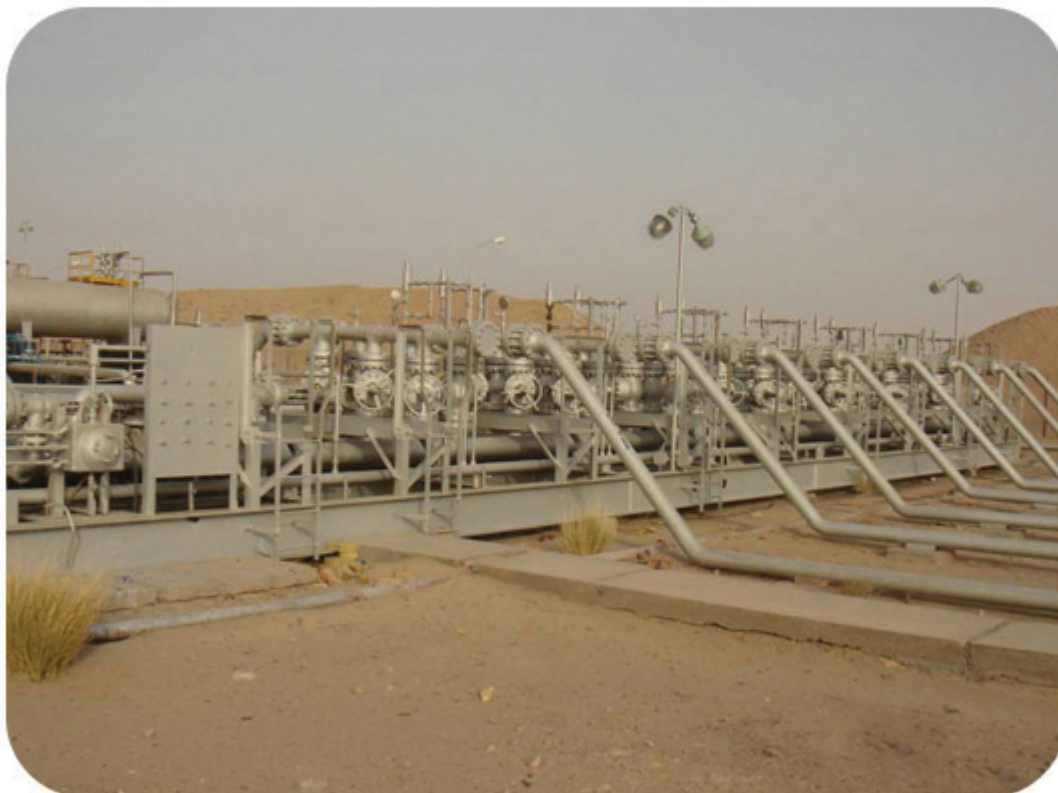
Image 6: Existing Manifold at Luhais Central - To Be Doubled In Size
