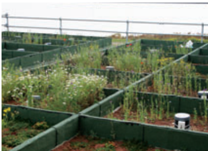
▲ Living roof at Barking Riverside, Barking, London Borough of Barking and Dagenham.
