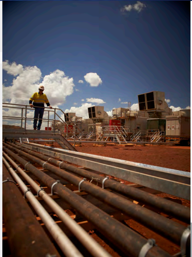
Solomon Power Station
