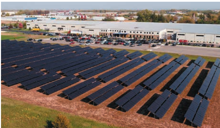
1.4MW solar array at Oshkosh distribution centre completed in 2022
