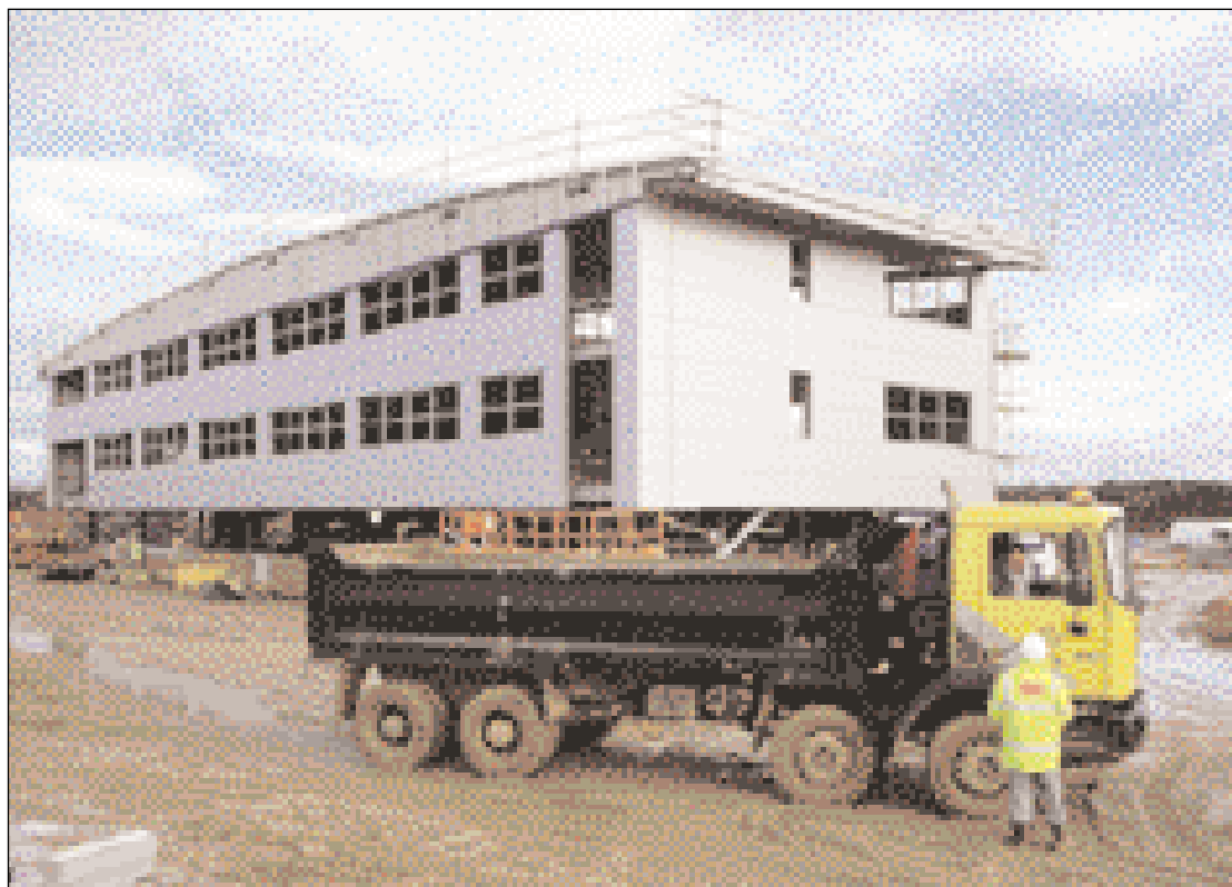
A 270,000 sq. ft. manufacturing, distribution and head office complex under construction for Duraflex at Tewkesbury, Gloucestershire. Completion due in 2004.
