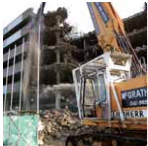
Multi storey car park Demolition of the multi storey car park underway in November 2004.
