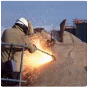
Site clearance Decommissioning of the former zinc smelter works, part of the site clearance programme.
