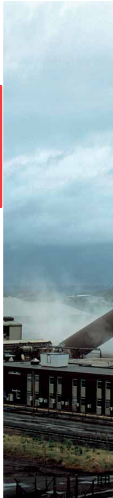
Demolition The toppling of the main chimney was completed in 2004, a highlight of the site clearance.
