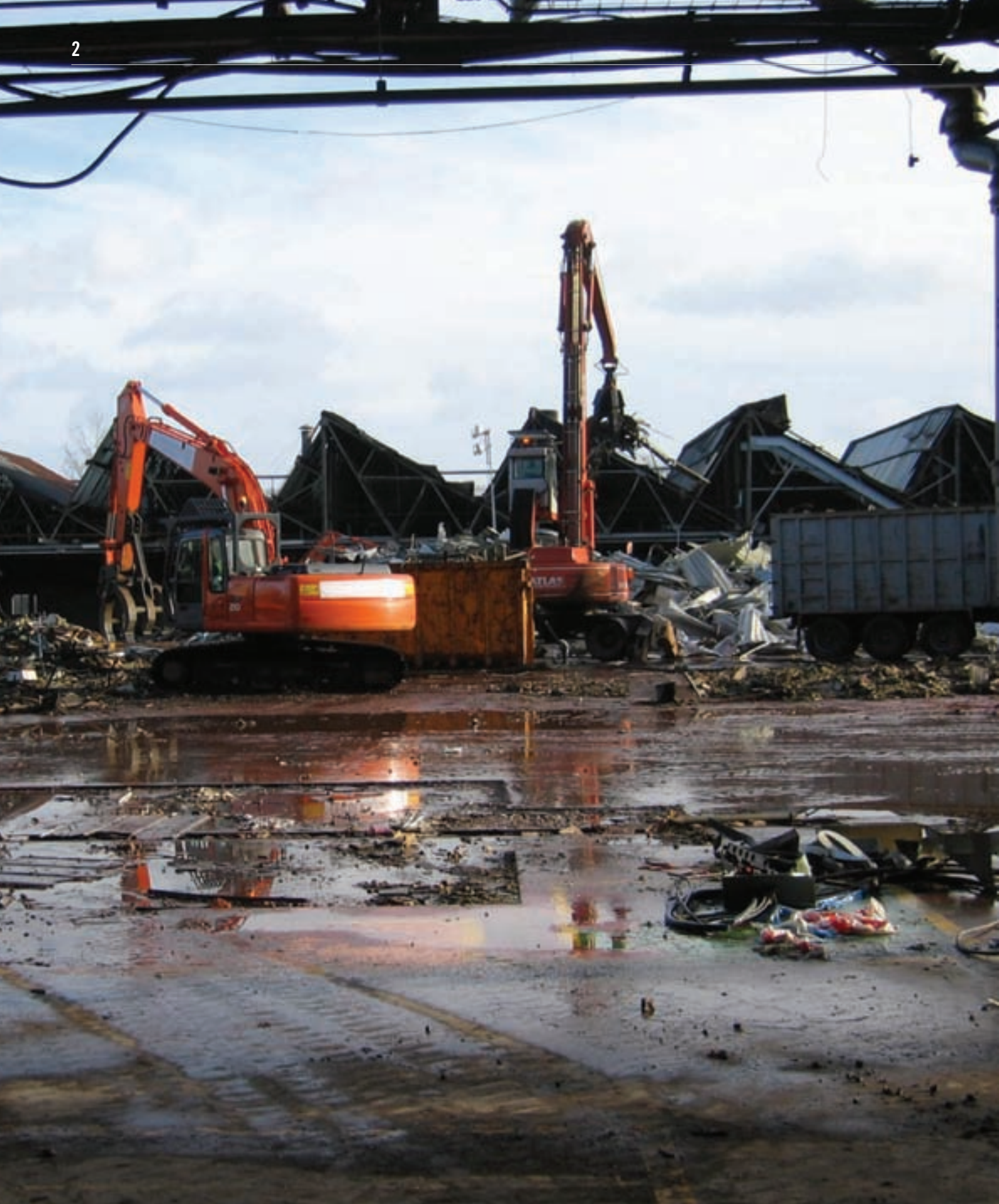
▲ LONGBRIDGE DEMOLITION IN PROGRESS. OVER 2M SQ FT OF REDUNDANT FACTORY SPACE HAS BEEN DEMOLISHED WITH OVER 90% OF THE DEMOLITION PRODUCTS SENT FOR RECYCLING OR REUSED ON SITE (A PARTNERSHIP PROJECT WITH AWM)
