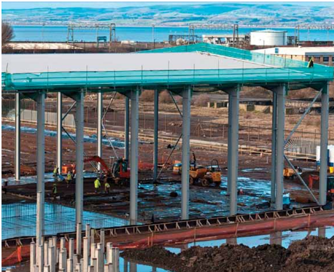
← The 300,000 sq. ft. waste treatment and recycling facility for New Earth Solutions at Access 18, Avonmouth.
