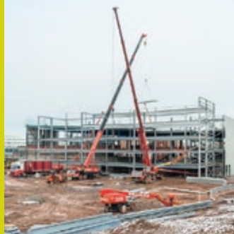
PICTURED RIGHT: 150,000 sq ft M&S store will be open for 2015 Christmas trading at Longbridge Town Centre, Birmingham.
