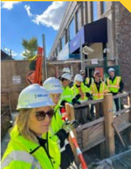
This picture has been taken at one of the site visits the Board conducted in New York in October 2022, where they learned about secant piles and jet grouting and met with local colleagues and divisional management.
