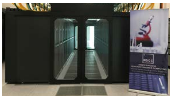
Singapore's National Supercomputing Centre
