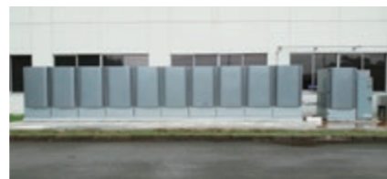
The fuel cell power generation system of Kumagaya Service Solution Center
