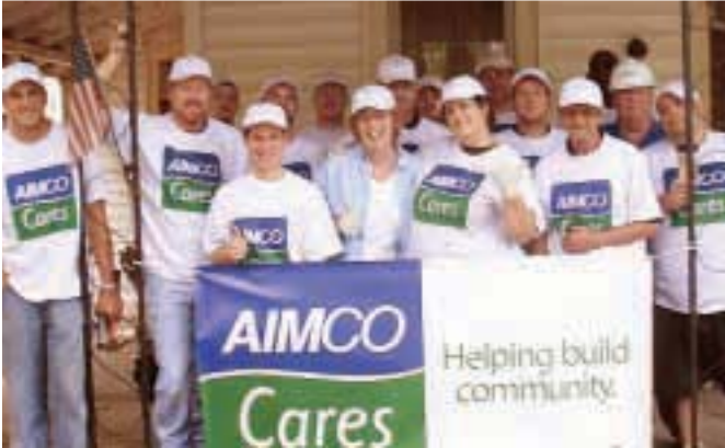
Aimco team members in Indianapolis volunteered to remodel a home for low-income seniors as part of the national Rebuilding Together program.
