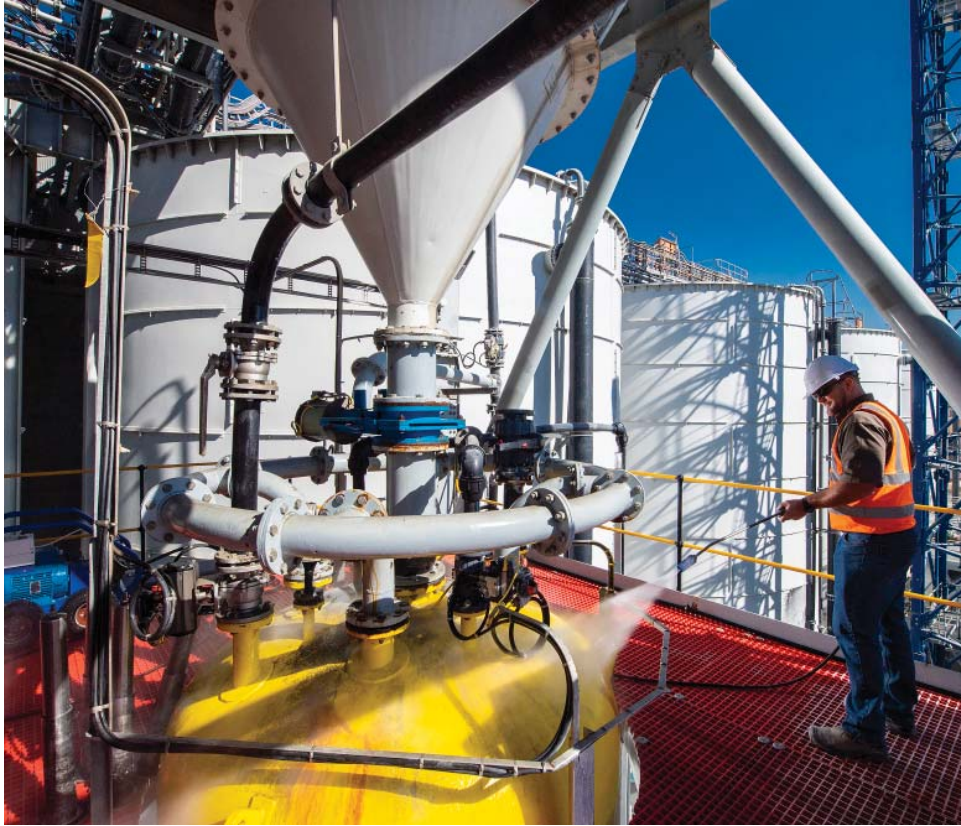
▼ Elikhulu plant – acid wash column
