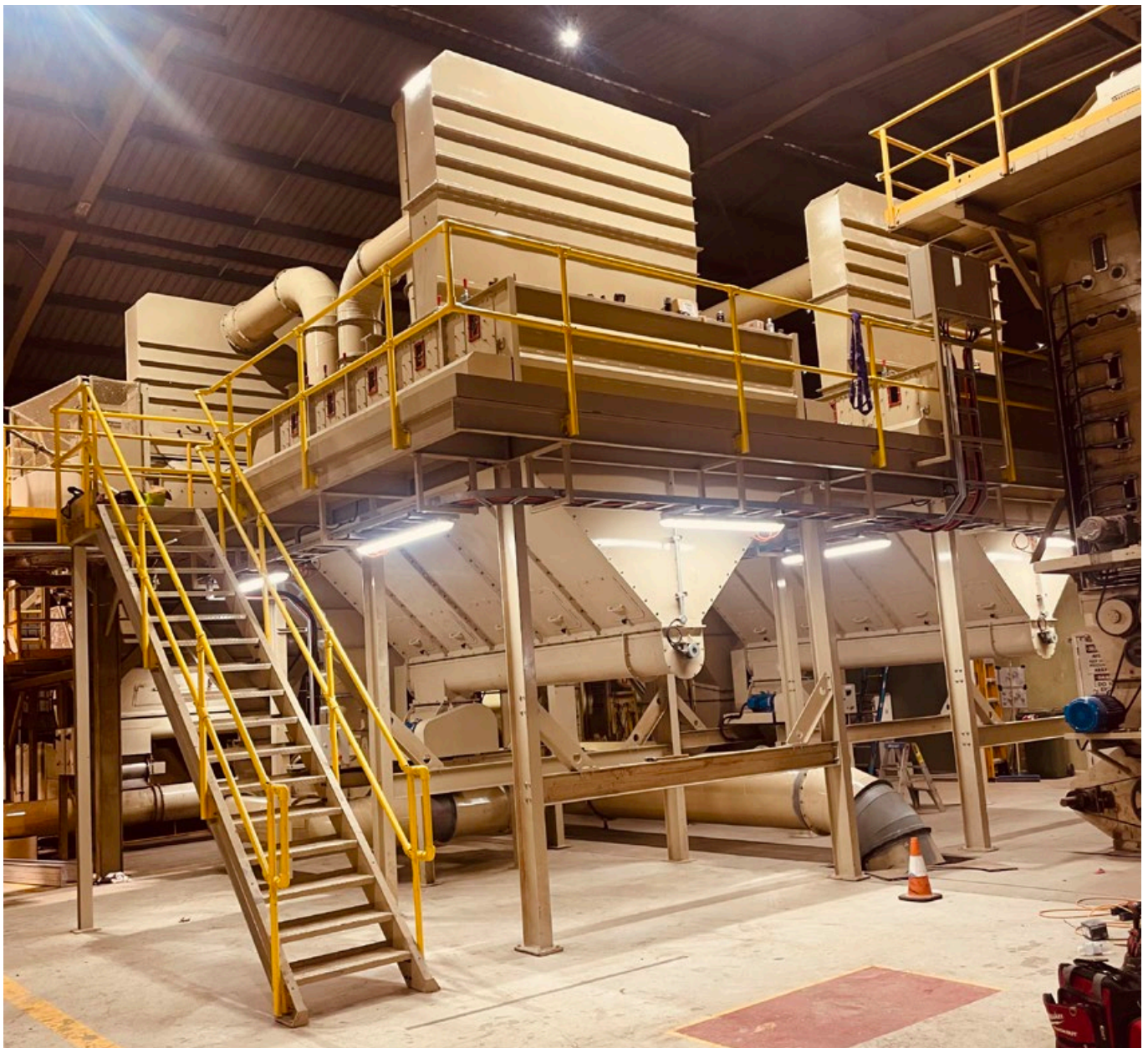
New drying and cleaning gin equipment at Merah North
