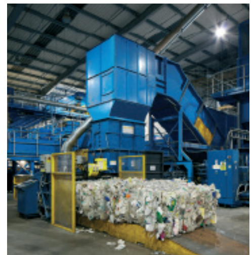
Viridor Polymers recycling facility, Skelmersdale
