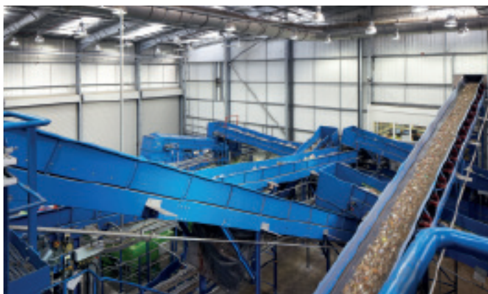
Materials recycling facility, Manchester
