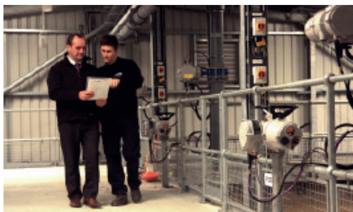
Water treatment works, Tottiford
