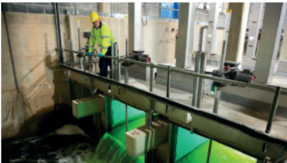
UV treatment at Waste Water Treatment Works, Brokenbury
