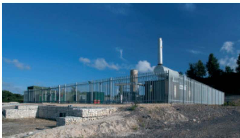
Landfill gas power plant, Dorset
