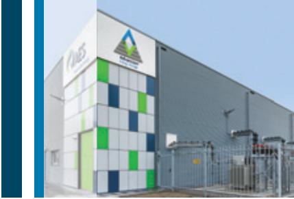
Advancion Energy Storage Array
