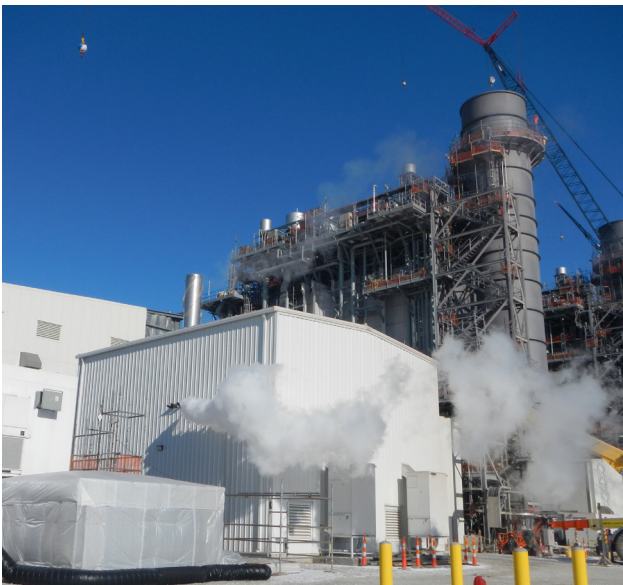
671 MW Eagle Valley (CCGT, Indiana-US)
