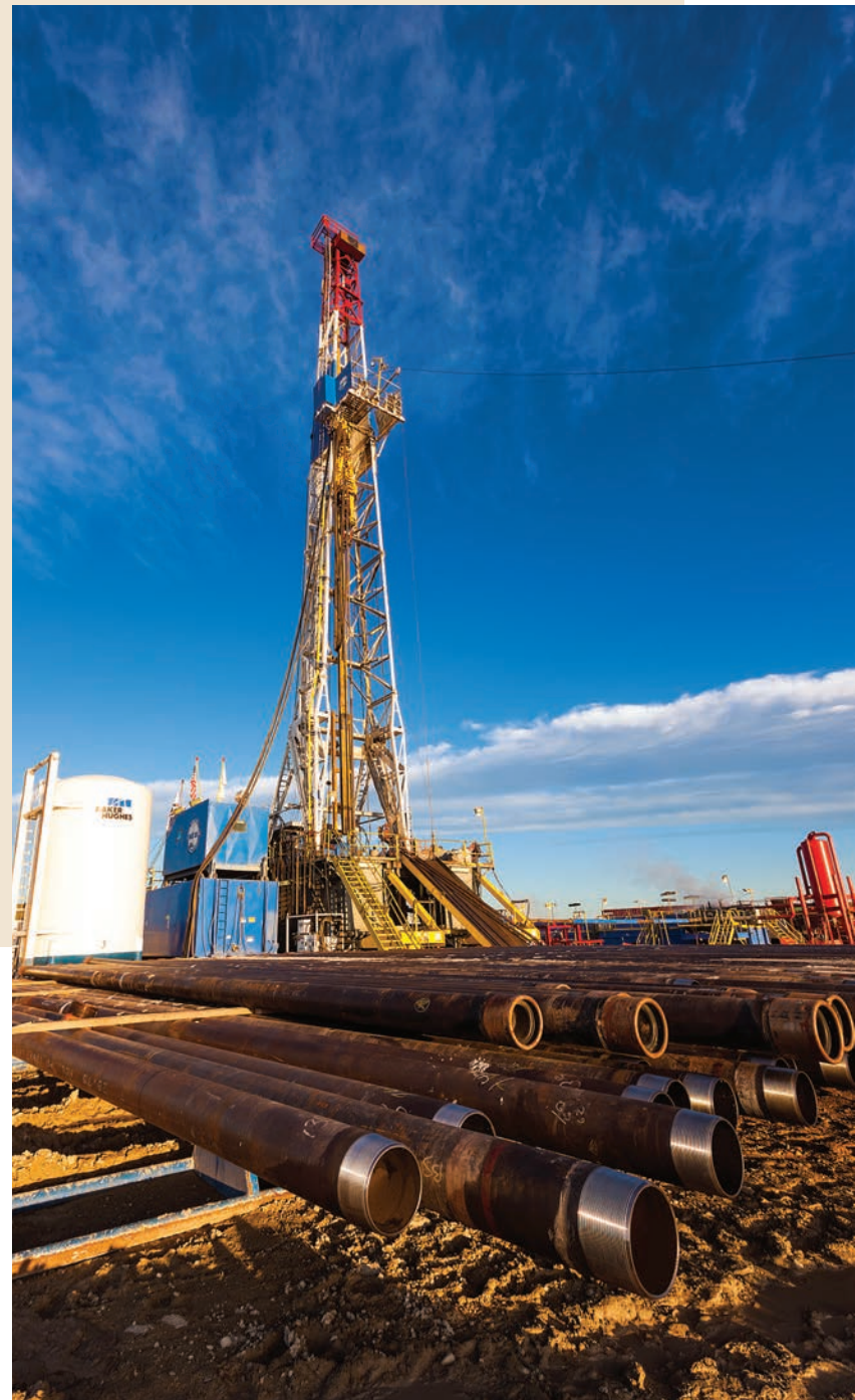
(RIGHT) Drilling operations on the Razor 271-2214B well at our Redtail Field in Weld County, Colorado.
