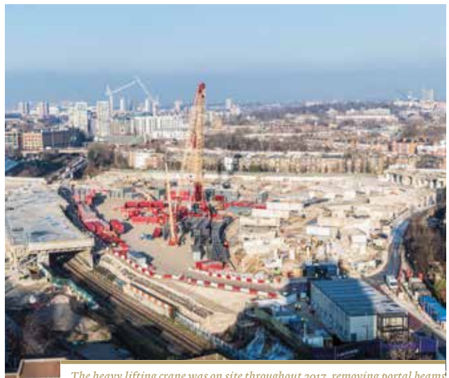
The heavy lifting crane was on site throughout 2017, removing portal beams from site to allow site preparation work to take place
