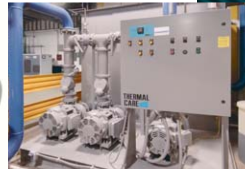
Thermal Care pump tank
