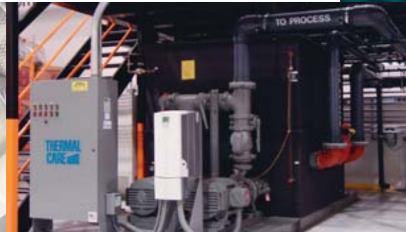
Thermal Care pump reservoir
