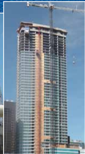
A Midwesco Mechanical project
