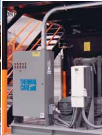
Thermal Care pump reservoir
