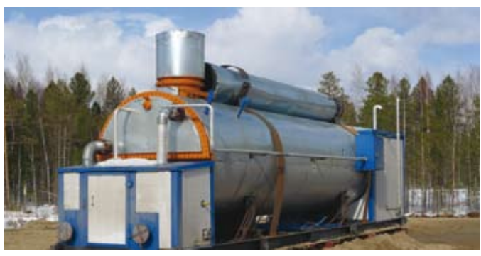
A heater which will be used in the oil processing facilities at Lineynoye.
