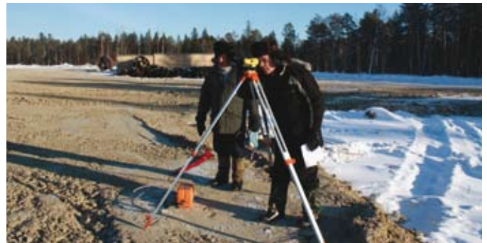
Survey work for the oil processing and storage facilities at the Lineynoye oil field on Licence 61.
