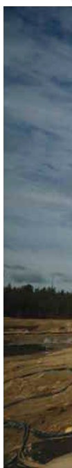
Pictures (from left to right): - Alexander Tarasenko, Shift Manager Stimul-T. - Fire water tanks under construction at Lineynoye Central Processing Facilities. - Gas powered piston generators at the Lineynoye oil field use associated gas for power generation.
