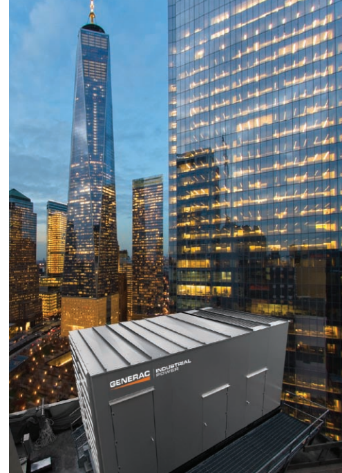
LARGE KW INSTALLATION
