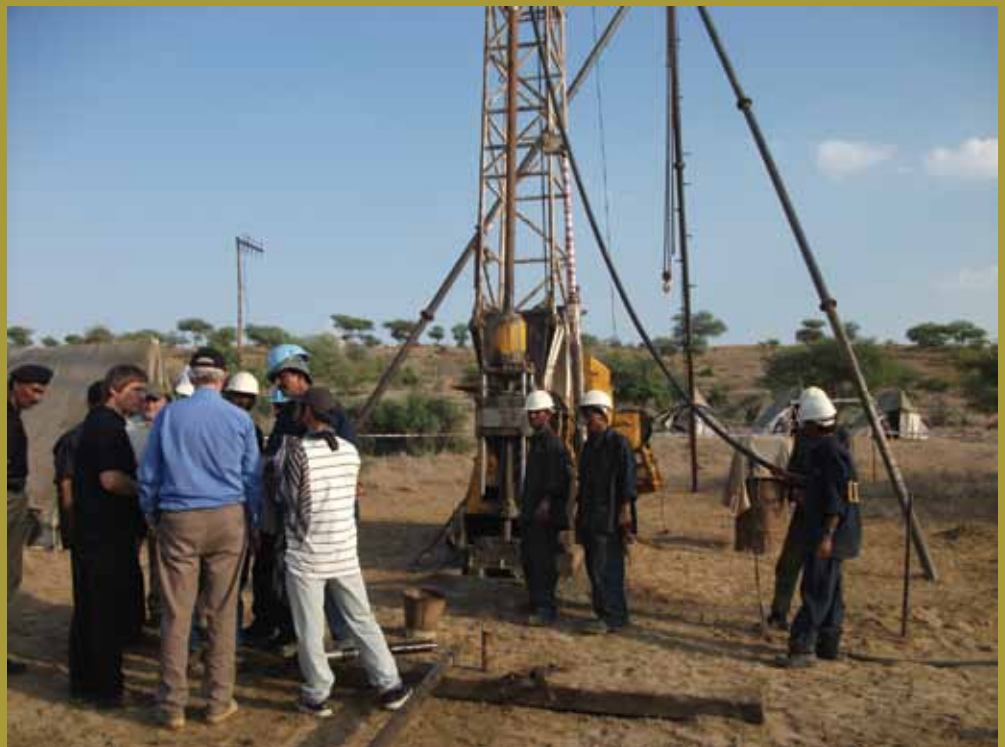
Geotechnical drilling at Block VI site overseen by Oracle Coalfields' independent consultants SRK Consulting and Dargo Associates, 13th October 2010
