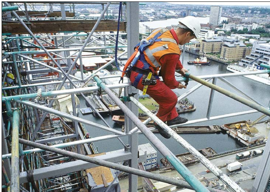
SGB's David Carter installs the scaffolding for a new office building in the heart of London's financial district. The task of ensuring a safe working environment begins well before the start of construction. Harsco's comprehensive services include pre-construction access design and on-site coordination throughout the project, matched by the industry's most complete range of scaffolding, forming and shoring equipment.
