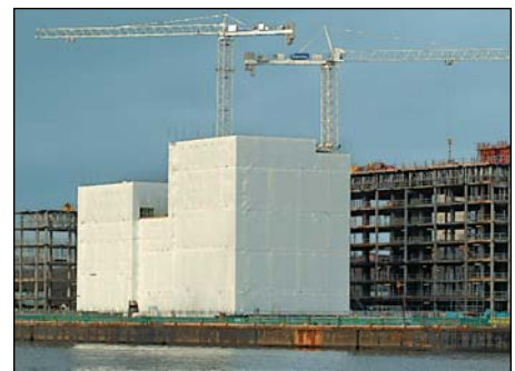
SGB's rental scaffolding is in wide use at this construction project in Glasgow Harbour, Scotland. Also included is SGB's new EnviroWrap shrink-cladding system which allows light inside during construction, but keeps weather out.
