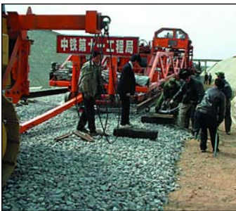
Harsco is supporting China's railway modernization and expansion initiatives with leading equipment like this New Track Construction train. With approximately 44,000 miles (71,000 km) of track, China's railway system is the third largest in the world, and the largest in Asia.
