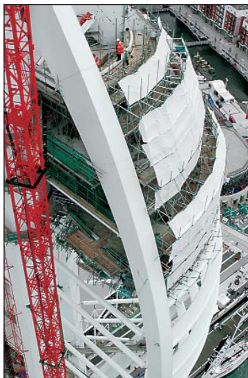
SGB has supplied scaffolding for the construction of the UK's new Spinnaker Tower in Portsmouth. When complete, this dramatic 170-meter tall landmark will provide spectacular views of the English Channel and surrounding area.
