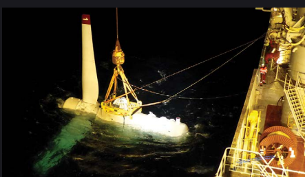
The 1.5MW AR1500 Atlantis tidal turbine being lowered into the water during installation
