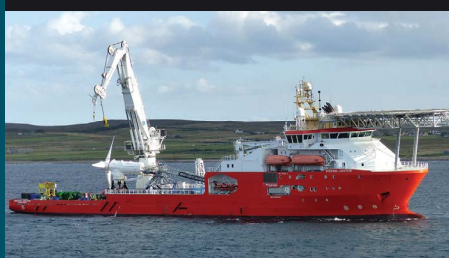
The Normand Jarstein DP Vessel installing the third 1.5MW Andritz Hydro Hammerfest tidal turbine
