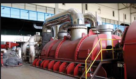
One of the 121 MW Turbines in the Uskmouth Power Station turbine hall
