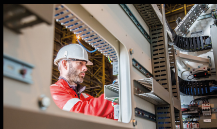
AR500 System Testing - Shop 1 Nigg Energy Park
