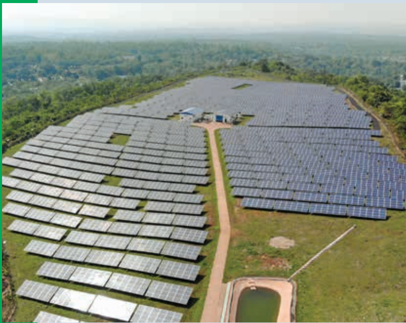
A 3 MW solar power plant at Noamundi iron ore mine
