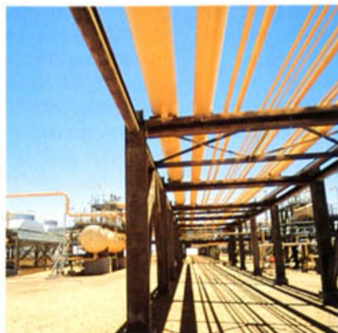
Ballera Gas Plant, south-west Queensland. $175 million will be spent on a major expansion of this facility and associated field development in 1996 and 1997.
